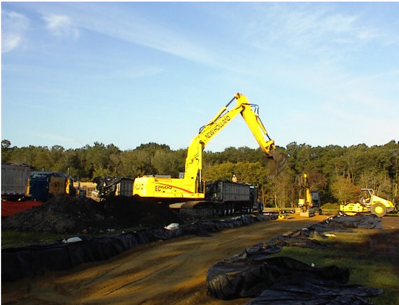
September 3, 2004 – View facing west-southwest of the North Corridor almost completely backfilled (post utility installation).
