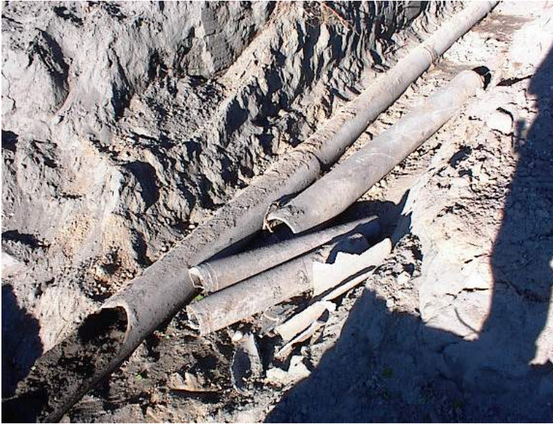
August 9, 2004 - Removal and replacement of crushed drain line through wetlands abutting western portion of McCoy Field.
