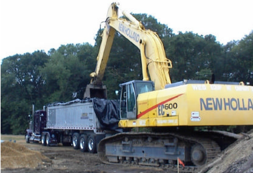
July 13, 2004 - Loading soil into pre-lined trucks and securing plastic sheeting on top of soil pile.
