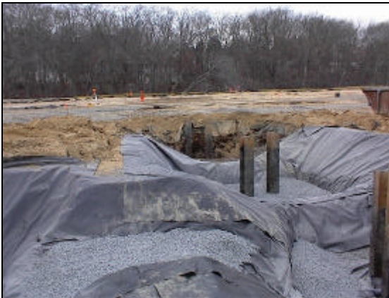
Photo 9: December 6, 2004 – Pile cap excavations, backfilled with crushed stone after lining, photo facing northwest.
