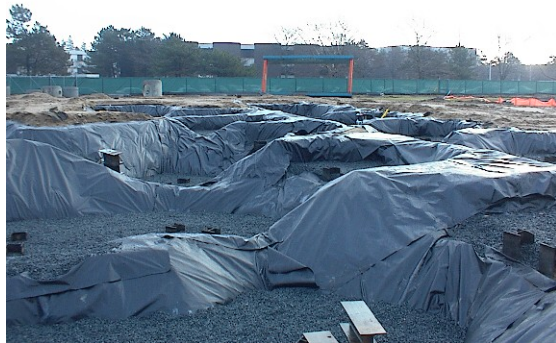
Photo 8: An example of an area of complete pile cap excavation (facing east).
