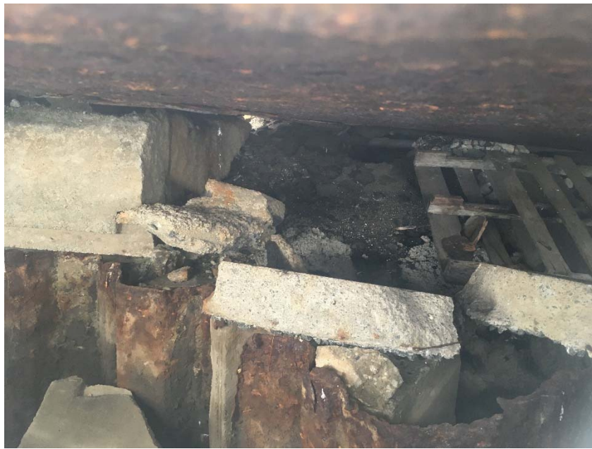
PHOTO 5 – VOID UNDER STEEL PLATE
