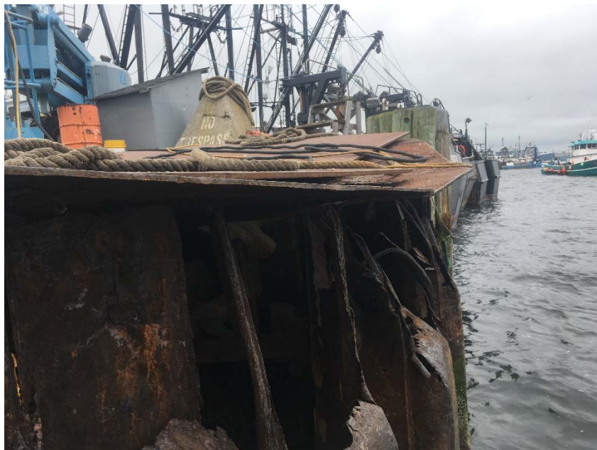
PHOTO 3 – SEVERELY CORRODED STEEL BULKHEAD
