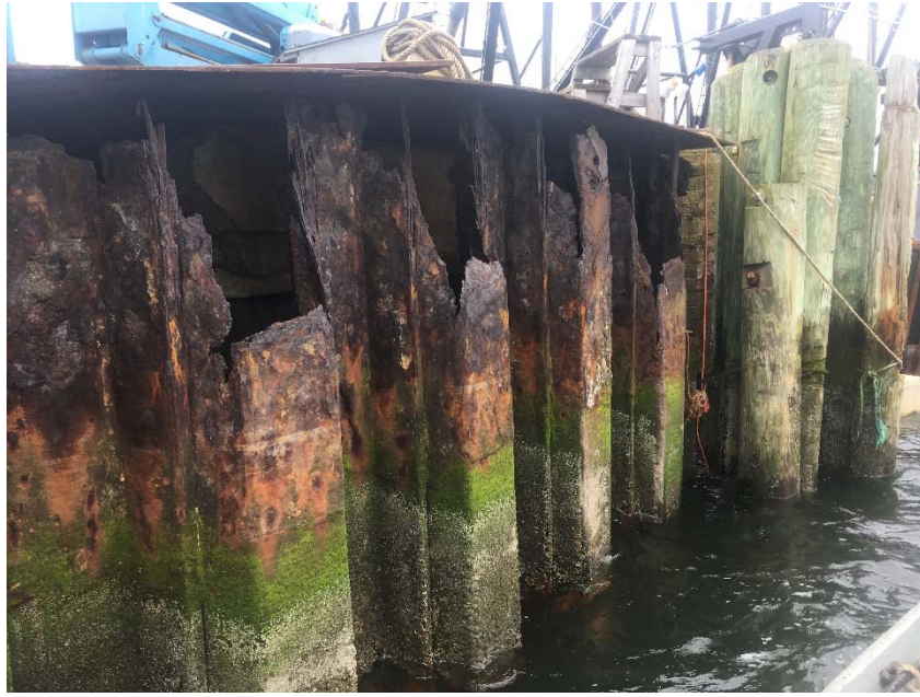
PHOTO 2 – SEVERELY CORRODED STEEL BULKHEAD
