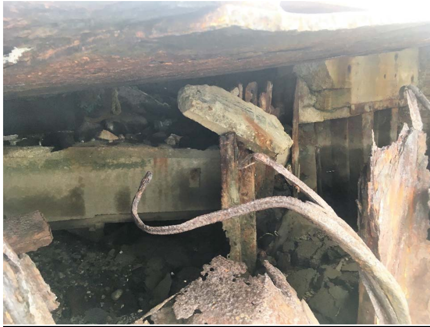
PHOTO 4 – VOID UNDER STEEL PLATE
