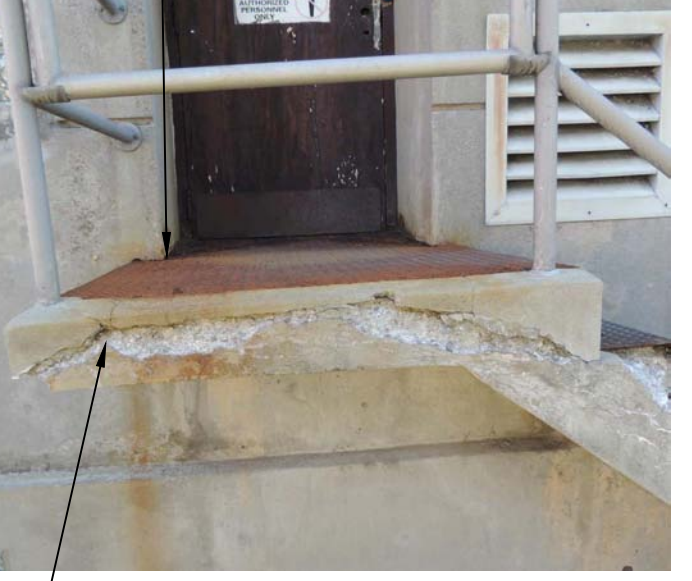
REMOVE EXISTING STAIR LANDING AND STAIR. REPLACE WITH NEW ENLARGED CONCRETE PLATFORM STRUCTURE TO SUPPORT GENERATOR PEDESTAL AND NEW CONCRETE ENTRY STOOP AND STAIRS. (PENDING)
