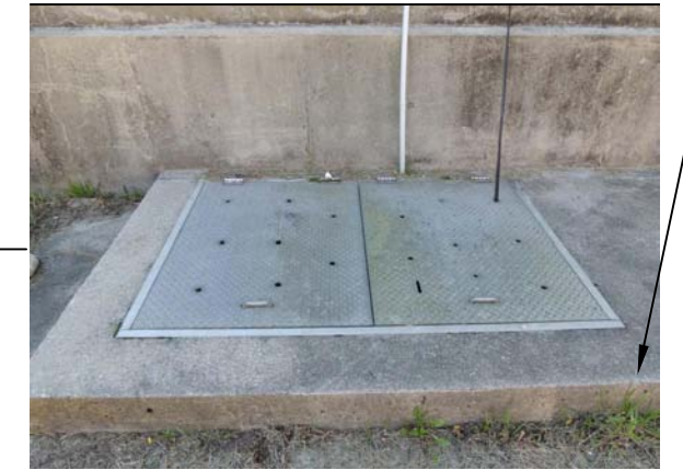
REPLACE EXISTING HATCH WITH FLOOD-PROOF HATCH AND MANWAY SAFETY ACCESSORY HARDWARE. (PENDING)
